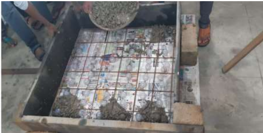
Figure 3.7 Placing of polypropylene balls in the centre of reinforcement & laying the concrete
