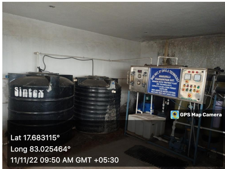
Water Treatment Facility
