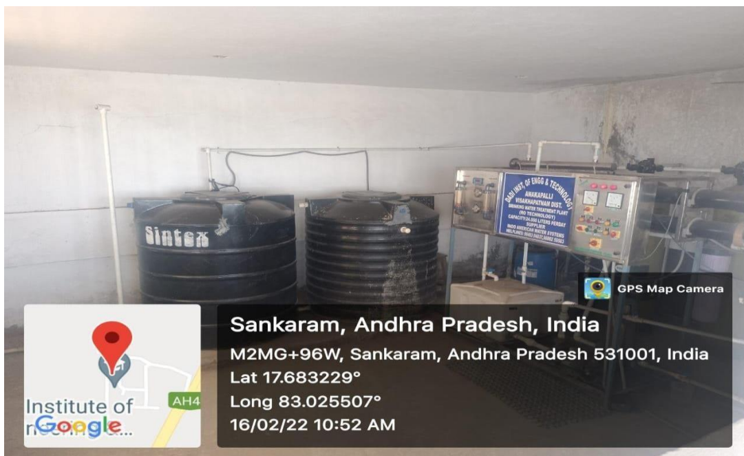
Water Treatment Facility
