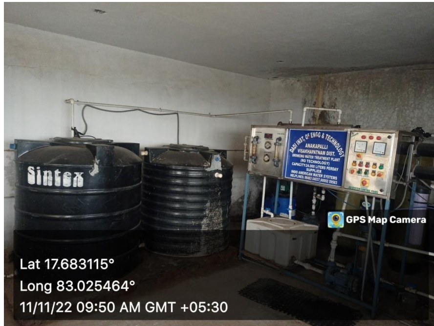
Water Treatment Facility
