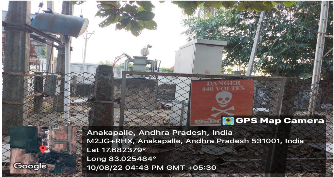
Transformer and Wheeling to the Grid at South-East portion of the Institution
