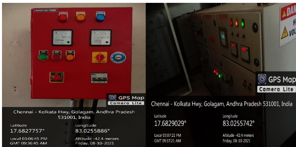
Devices installed for wheeling to the Grid
