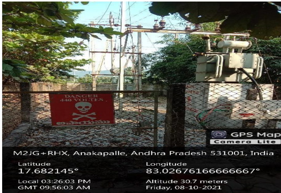
Transformer and Wheeling to the Grid at South-East portion of the Institution
